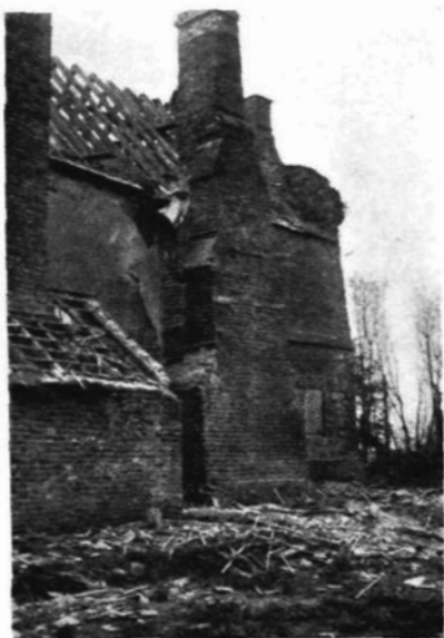
FIG. 1. HILLE'S COURT, ASH. Great chimney stack at back of house during demolition. April, 1940.
